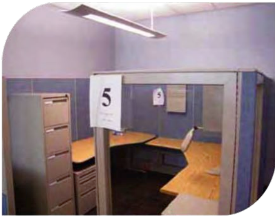
In networked lighting control, the goal is distributed points of intelligence, which includes smart dimming ballasts connected to smart switches.
